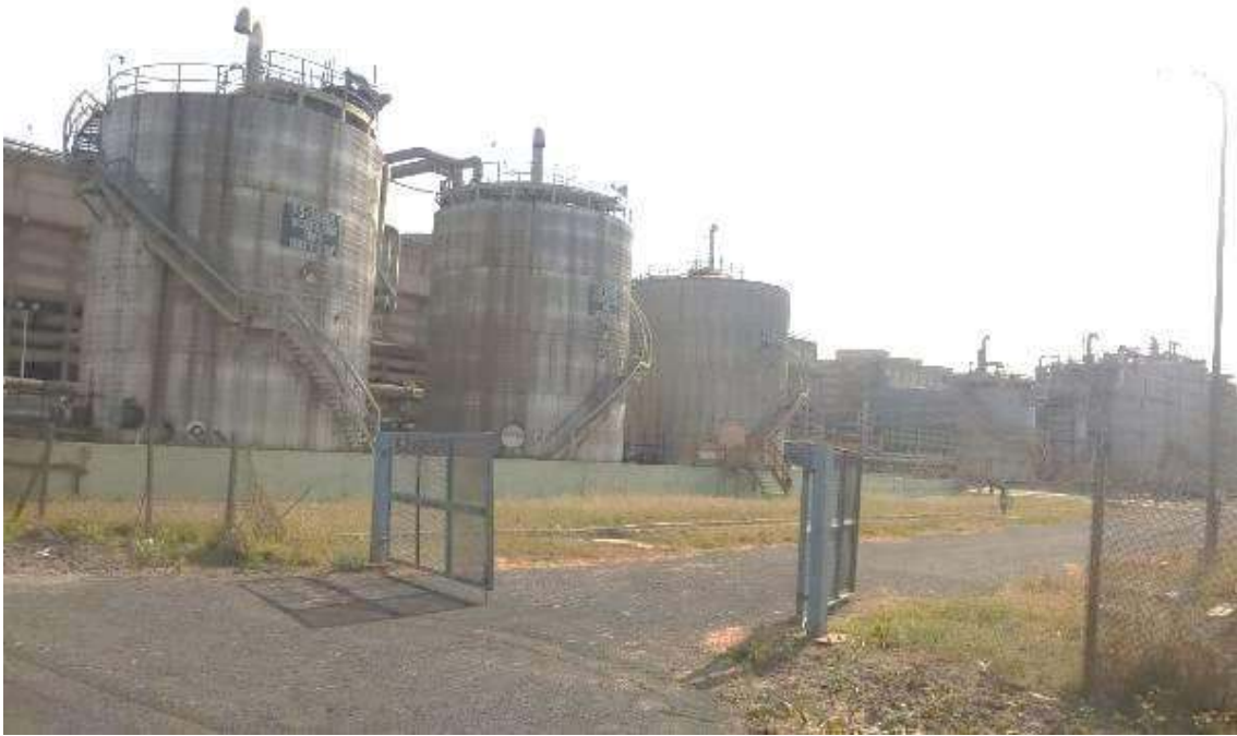
Photograph of PTA Storage Tanks
