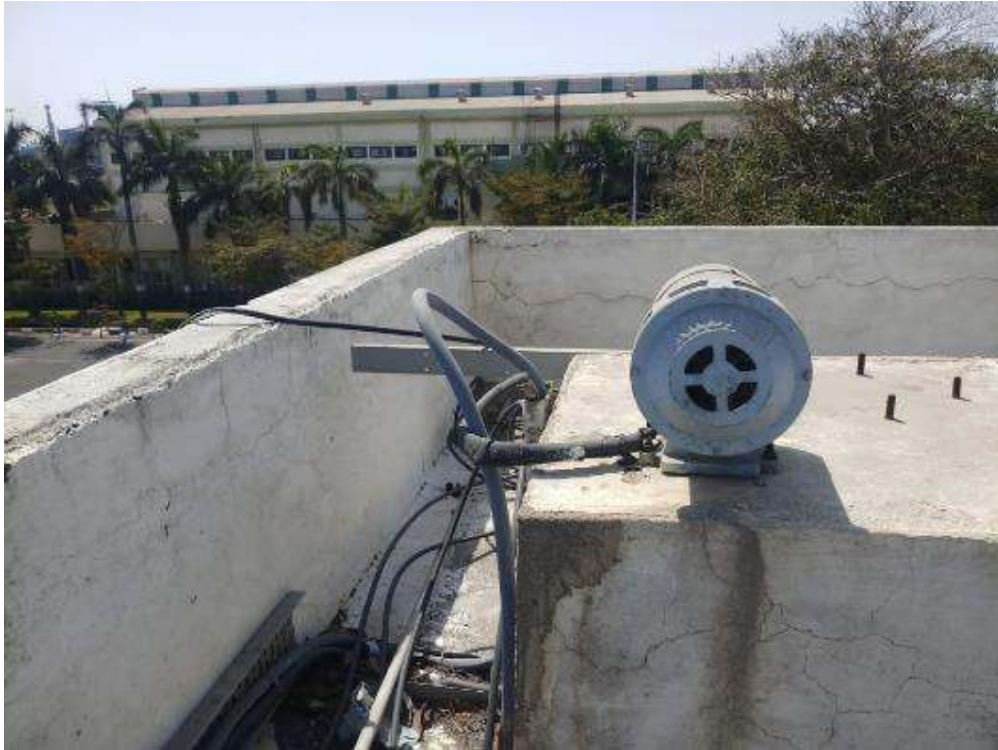
Photograph of Siren installed at SSM Building
