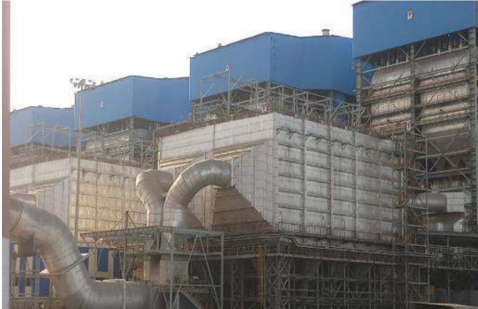
ESP's Installed at CCPP
