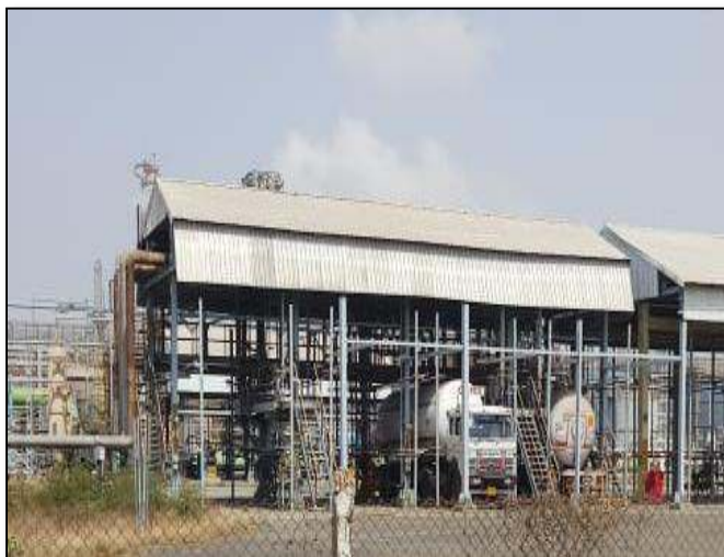
Loading Arms at Tank Farm
