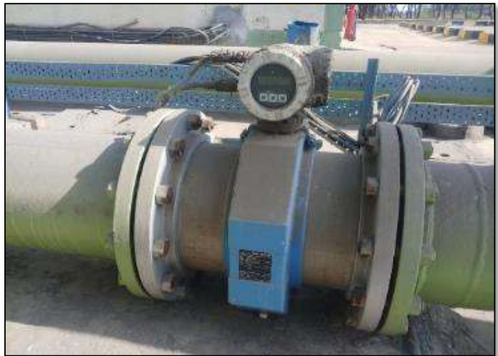
Flow Meters installed at ETP outlet
