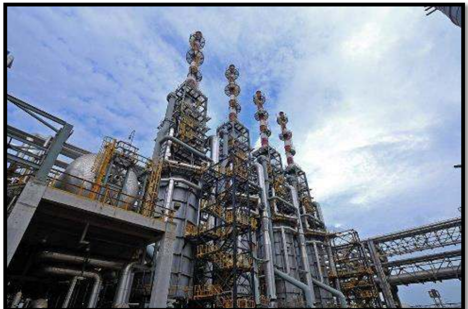
Stacks attached with HTM Heaters in PET Plant
