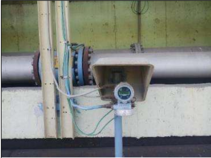
Flow Meters installed at ETP inlet
