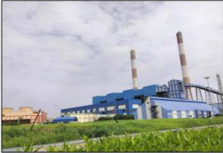
Stacks (Ht 220m) attached with Boilers
