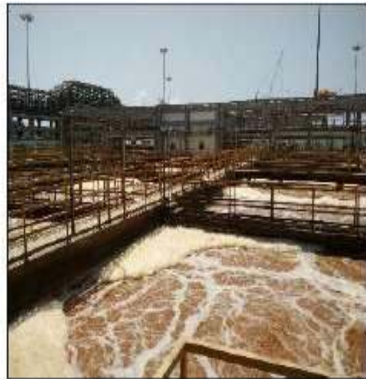
MBR Aeration Tank
