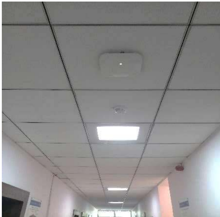
Photograph of LED lighting in offices
