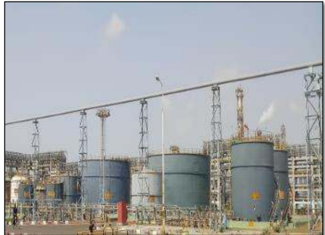
MEG / DEG Storage Tanks
