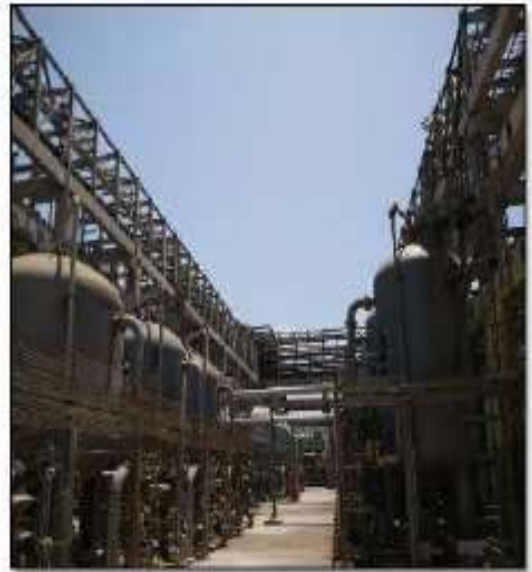
MEDIA FILTRATION SYSTEM
