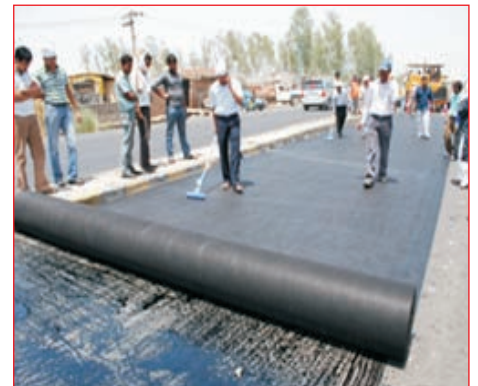
Govt of West Bengal & Arunachal Pradesh have included Geosynthetics in their SOR for Roads & River bank protection.
