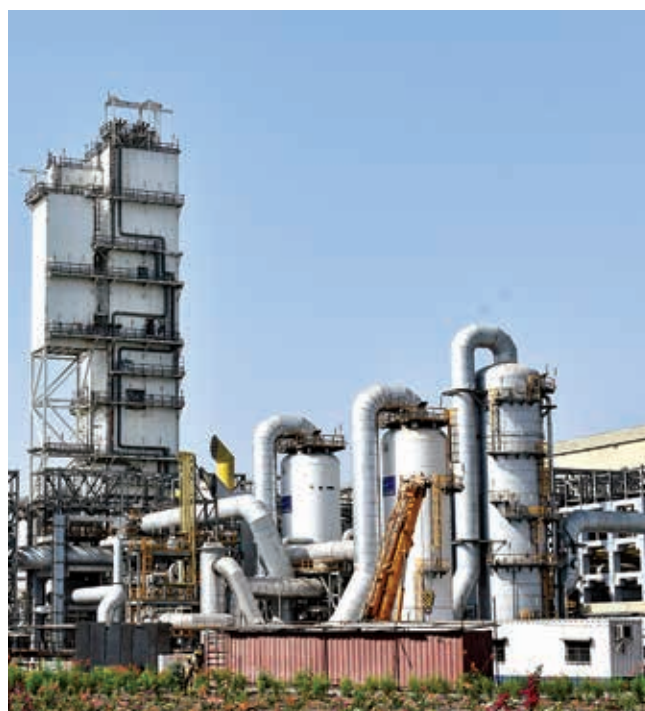
Gasification – Air Separation Unit
